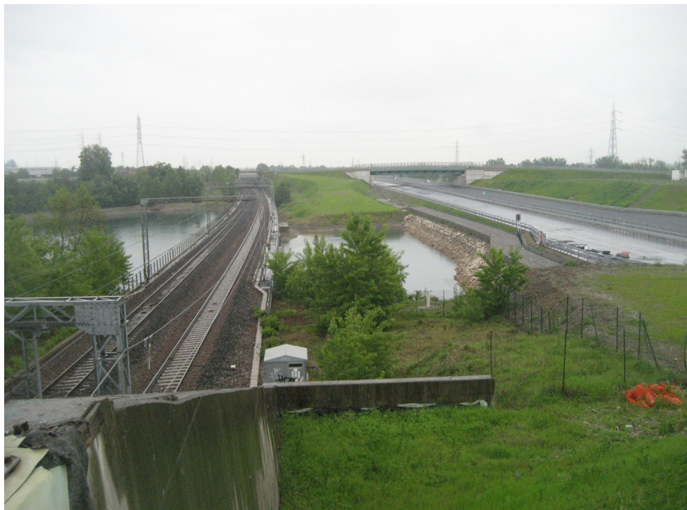
Fig. 4 – The Albignano Quarry at Truccazzano, with some environmental mitigation works in progress. Photo by G.P. Scaratti, May 2014.
