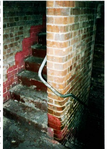
This stairwell led to the Boiler Room, deep underground at the ABC Portsmouth. Note the rounded bricks edging the staircase. Most architects and builders wouldn't be so thoughtful nowadays!
