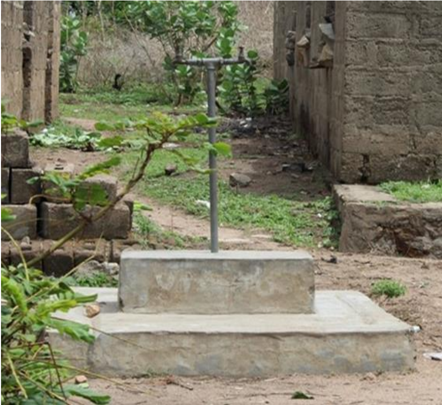
Figure 6-1: A public standpipe in Igànná . Source: Lead author
