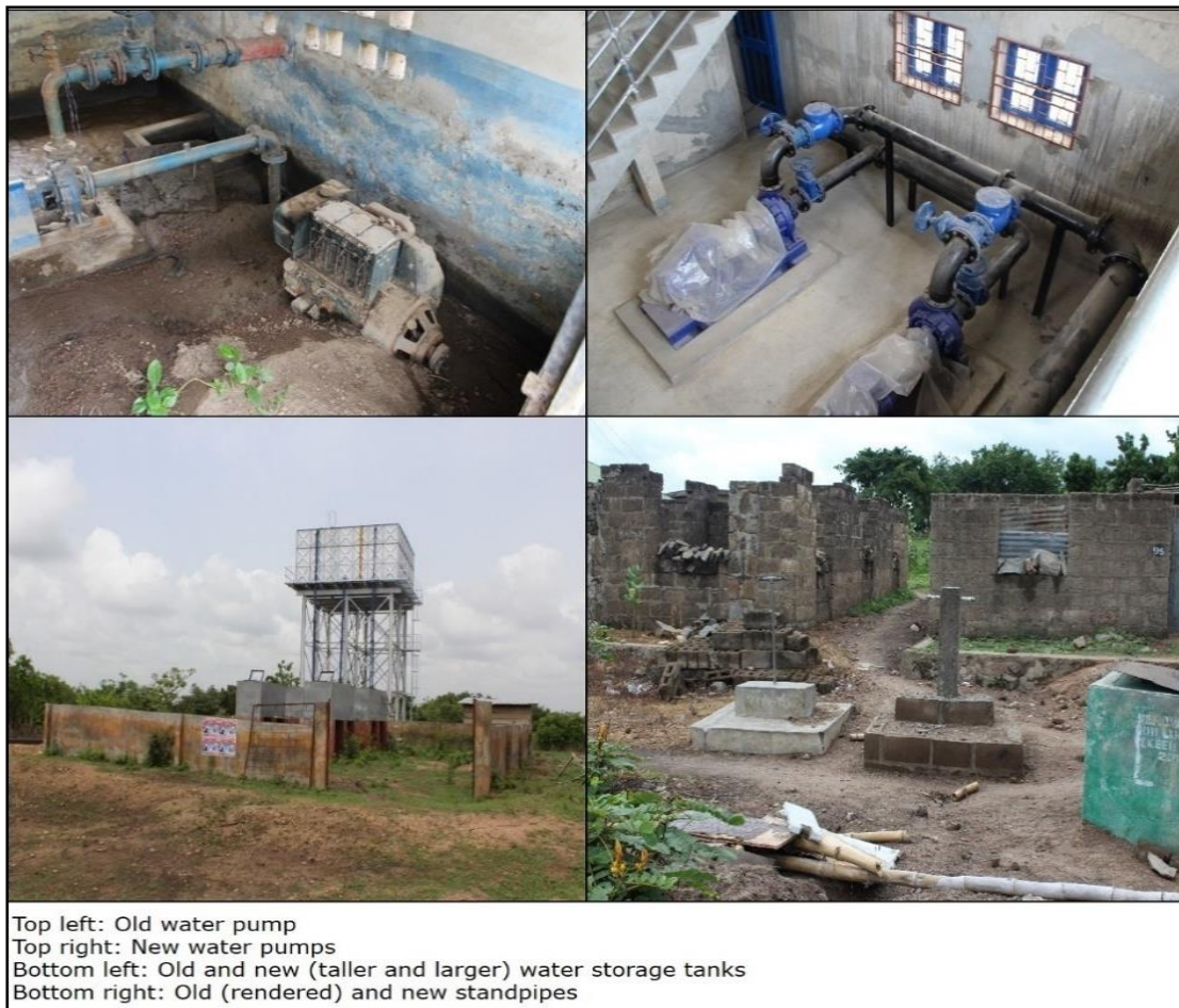
Figure 5-9: Old (constructed 1985) and new (constructed 2017) pumps, storage tanks, and standpipes. Source: Author
