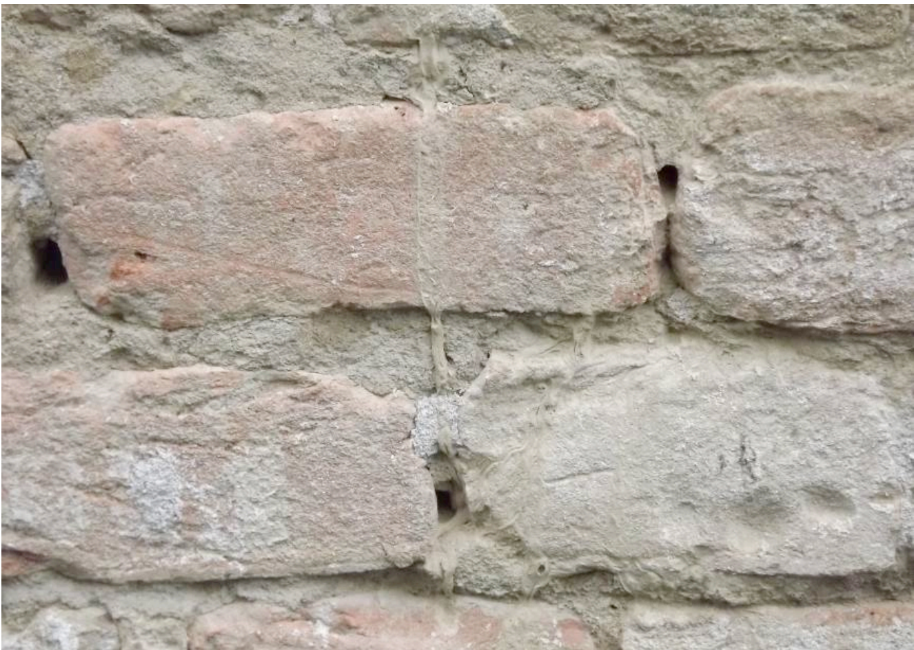
Figure 1. Detail of an earthen mortar masonry and the dripping of the earthen mortar, palazzo Magio Grasselli.
