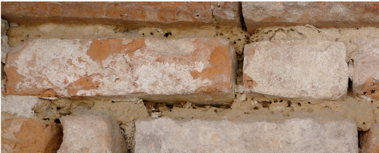
Figure 2. Decay of earthen mortars in palazzo Magio Grasselli
