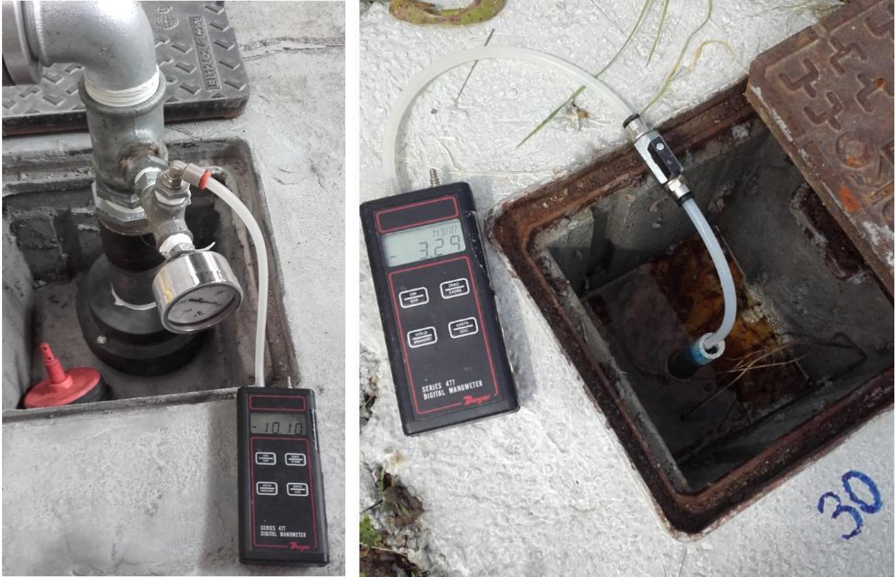
Examples of vacuum measurements at wellhead (left) and monitoring point (right)
