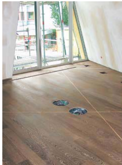
The intelligent floor structure incorporates heating and cooling capabilities
